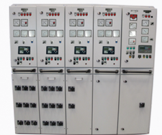
Main Switchboard & Marine Cables
